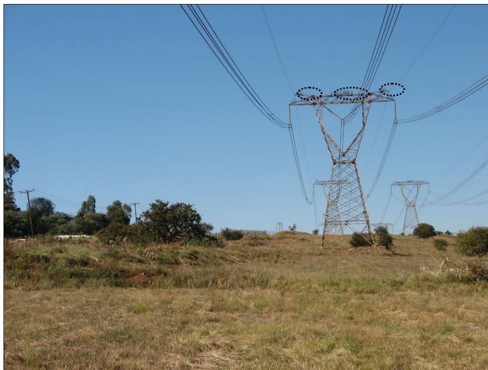
Figure 9: Bird guards (‘spikes’) fitted to a self-supporting tower.
